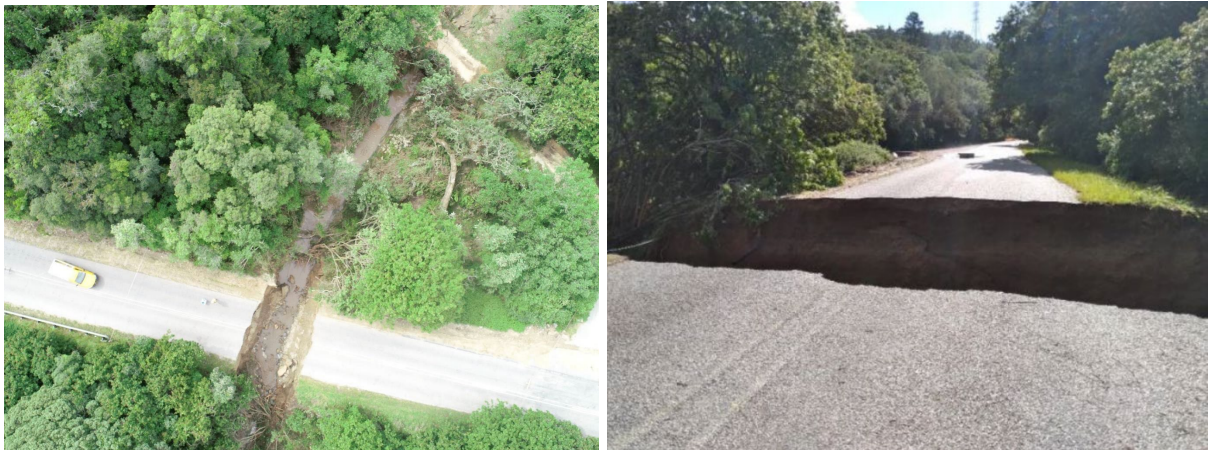
Figure 1: showing the damaged road.
