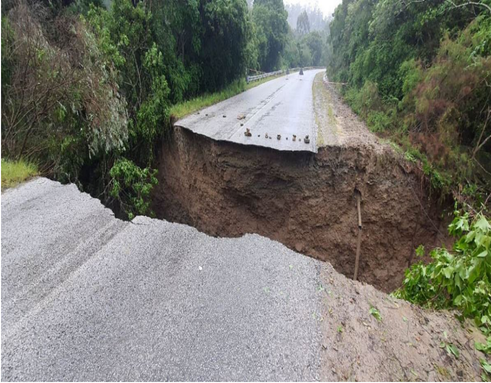
Figure 1: Slip failure, Armco washed away
